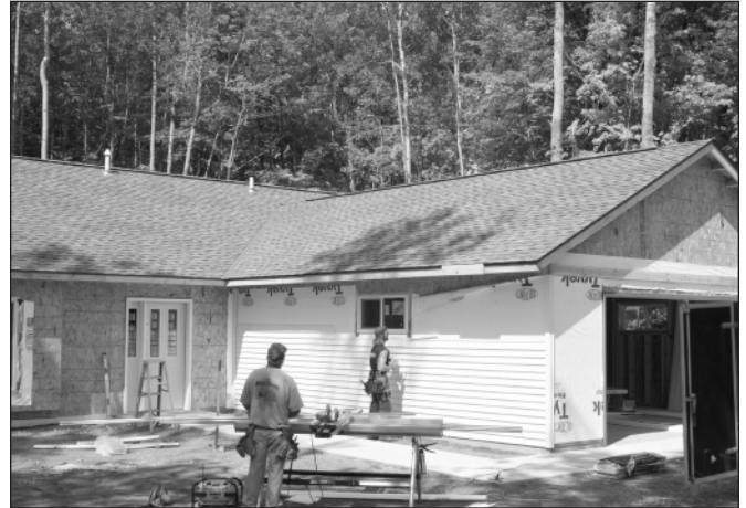
Since 1991 the Mille Lacs Band has built nearly 400 new homes and renovated many existing homes.
